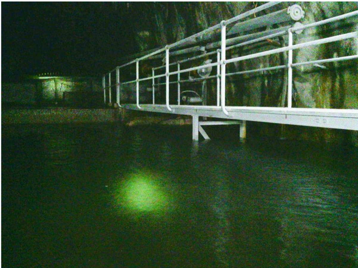
The walkway over the weirs just inside the 30m wall of the drift. The weirs collect water and silt, allowing the water to discharge from the weirs, and the silt to settle.
