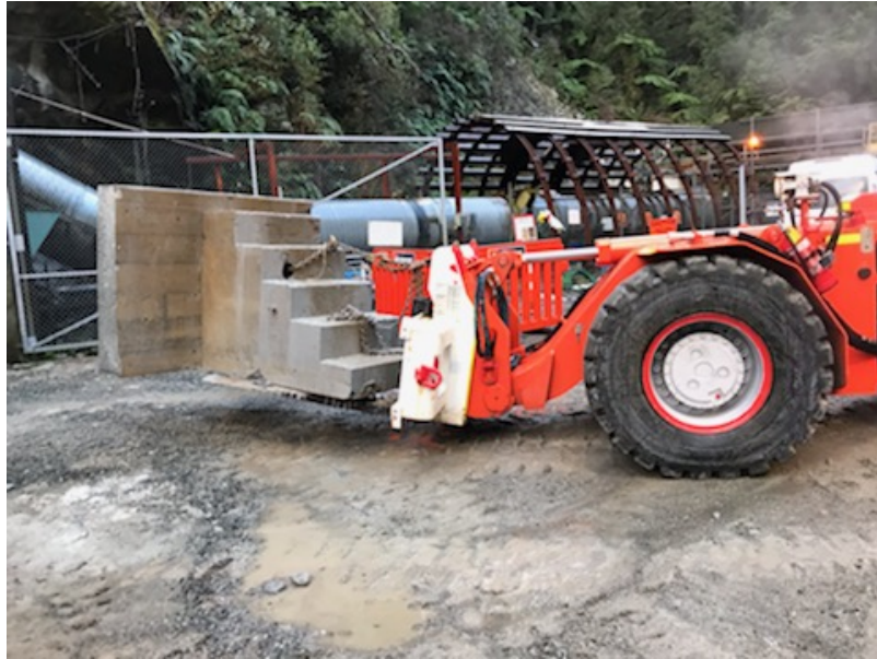
Steps to the walkway over the two weirs are removed from the drift.
