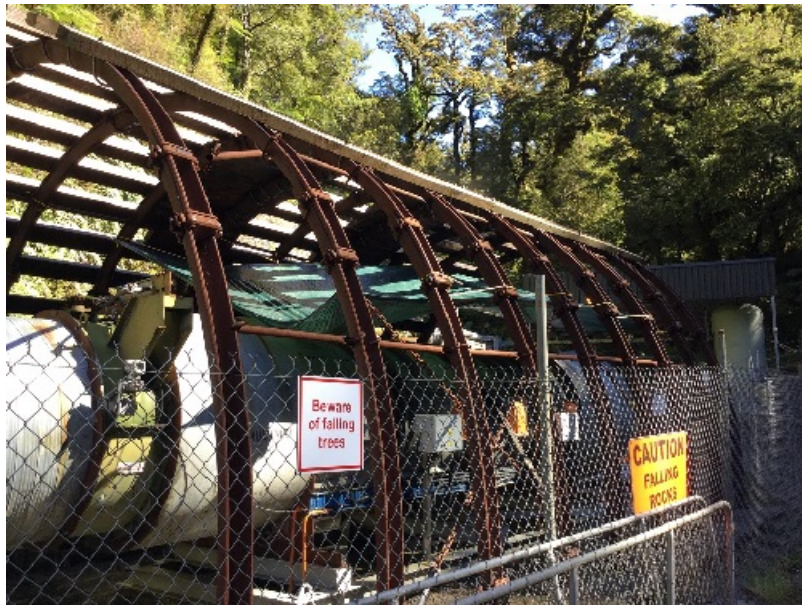
The main fan at the portal area.
